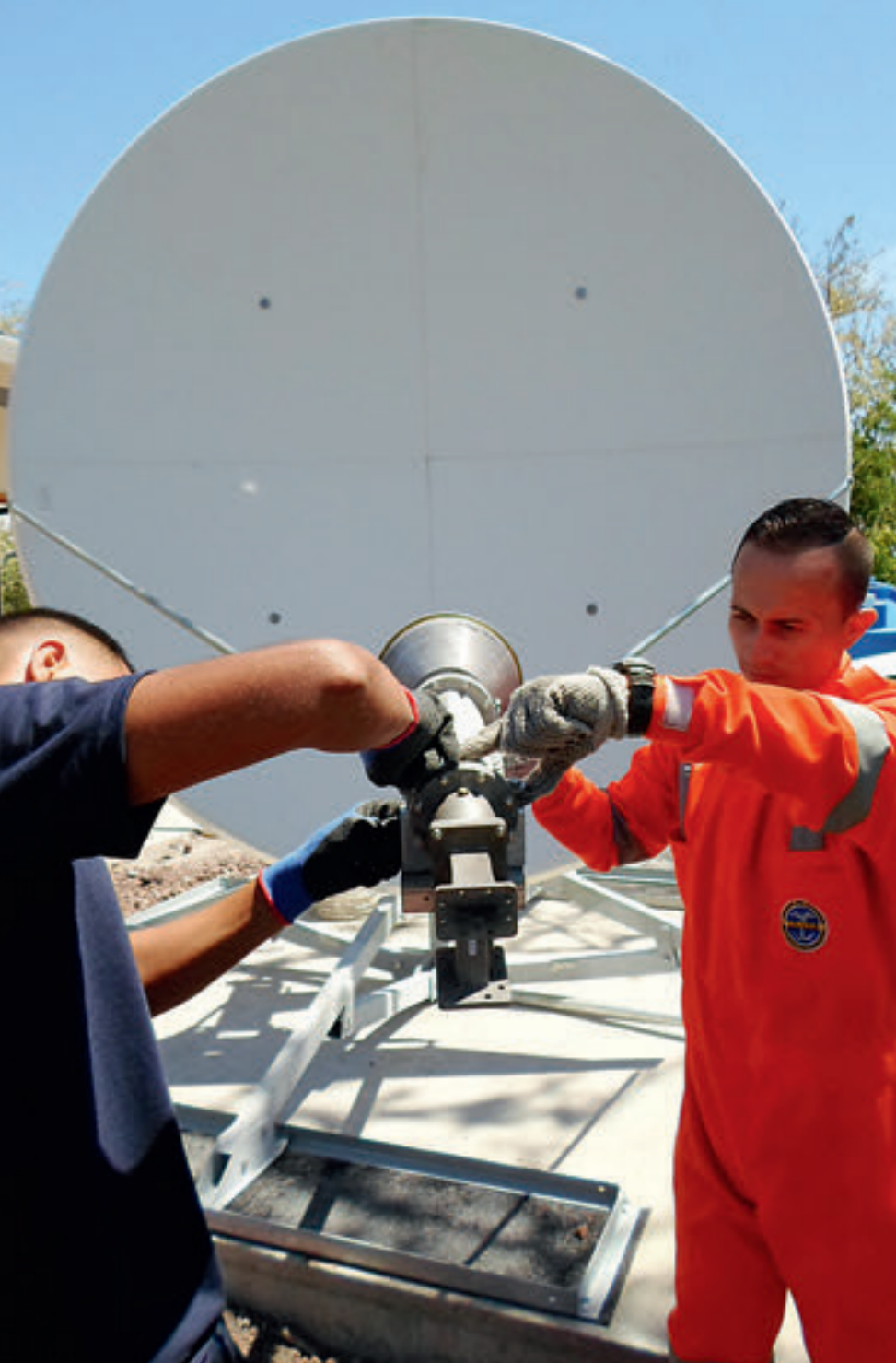
Top: Installation of GCI III on the roof of the Vienna International Centre. Bottom: GCI installation at infrasound station IS20 (Ecuador).
