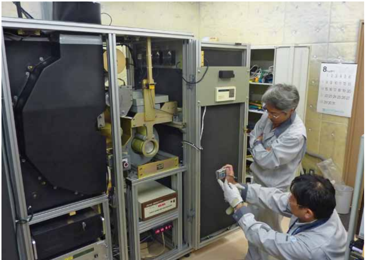
Operators verifying the installation of the detector system at radionuclide station RN38, Takasaki, Japan.
