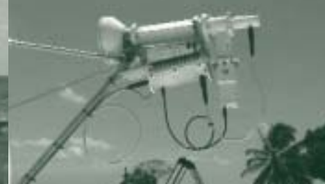
RADIO FREQUENCY POWER AMPLIFIER AT COCOS ISLANDS RADIONUCLIDE STATION, AUSTRALIA
