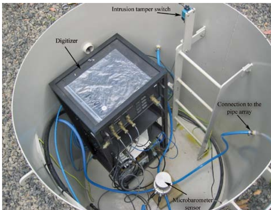
INSIDE OF AN INFRASOUND EQUIPMENT VAULT, INFRASOUND STATION IS04, SHANNON, AUSTRALIA
