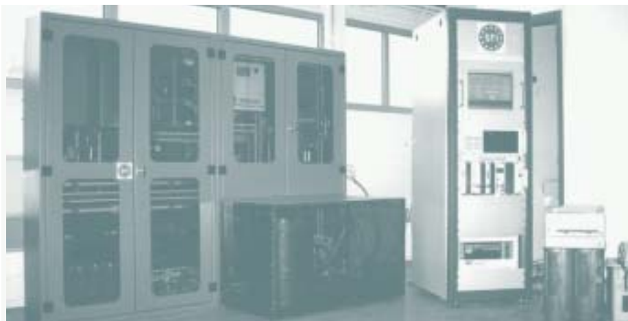
NOBLE GAS SYSTEM DEPLOYED AT RADIONUCLIDE STATIONS RN27 IN PAPEETE (TAHITI)
