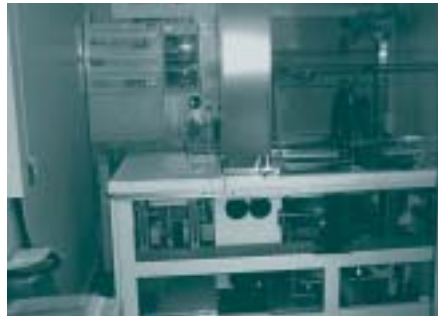
EQUIPMENT FOR FULLY AUTOMATIC SAMPLING AND ANALYSIS OF AIRBORNE RADIONUCLIDES, CTBT RADIONUCLIDE STATION SEP 63 IN STOCKHOLM (SWEDEN)
