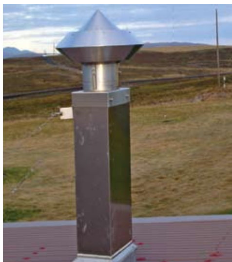
AIR INLET OF AUTOMATIC RADIONUCLIDE STATION, RN34, REYKJAVIK, ICELAND
