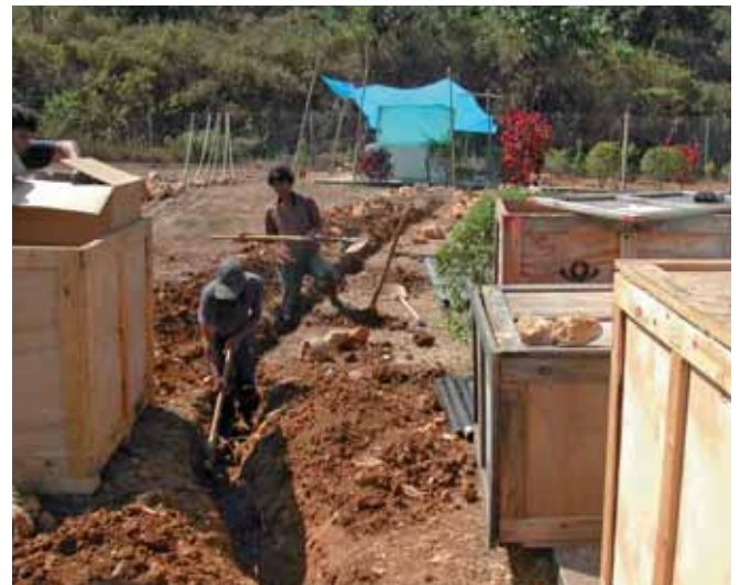
DIGGING A TRENCH FROM THE SENSORS TO THE CENTRAL RECORDING FACILITY, AUXILIARY SEISMIC STATION AS44, KAPPANG, INDONESIA
