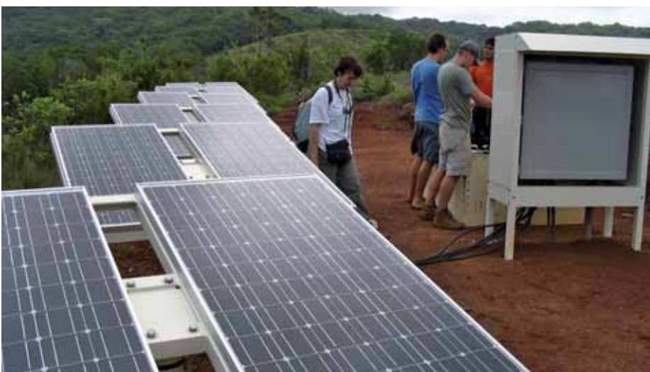
CENTRAL POWER SITE WITH SOLAR PANELS, IS39, PALAU
