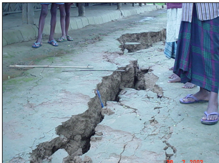
2003: Long crack along River, Kolabunia
