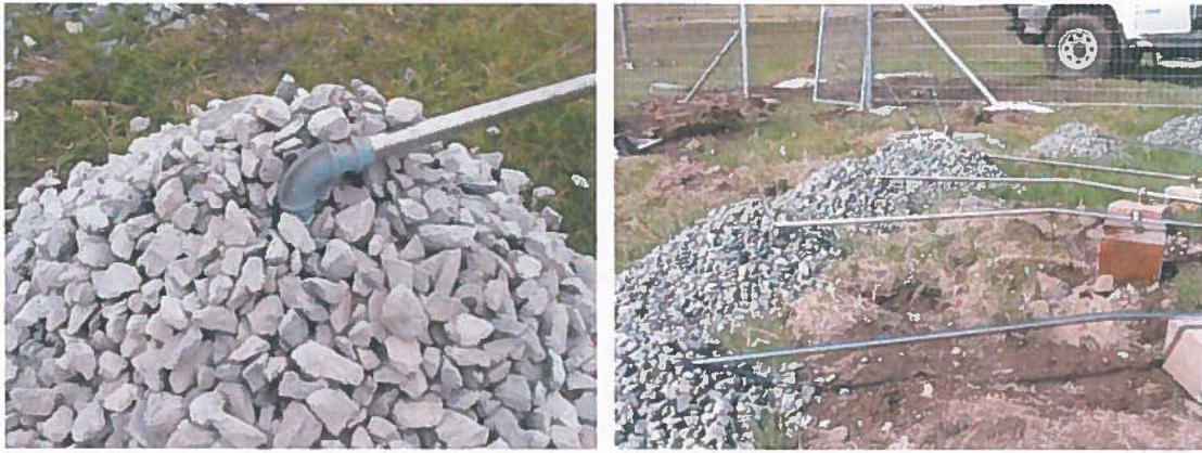
Figure 4: Inlet ports covered by gravel (photos taken during the installation of the Station)
